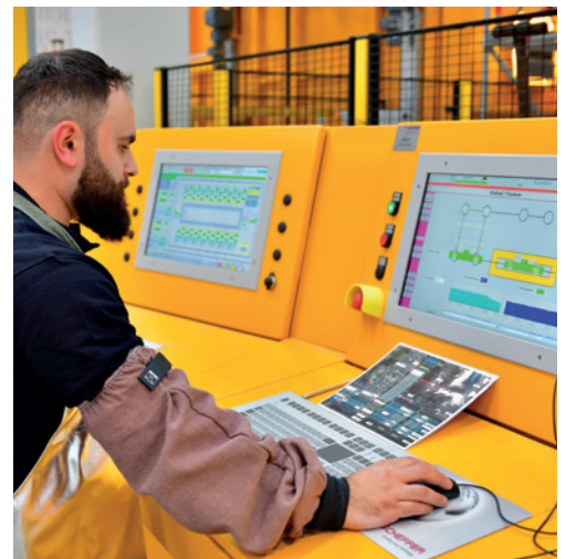
Digital control system
