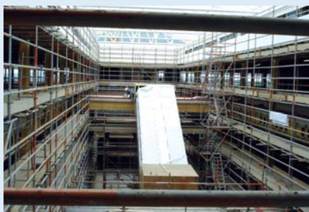
A view of the internal atrium during building work which has an apex of some 17.5 metres
