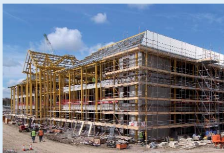
The new Morrison's Headquarters in Bradford during construction that gains from Layher's Allround® system
