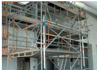
The new system is simply located to provide enhanced safety as a scaffold structure proceeds
