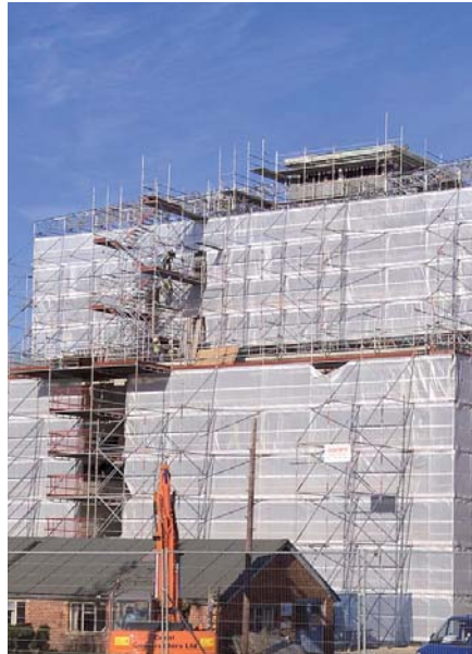
Comprehensive scaffolding at the Grade I structure in Farnborough despite tying-in restrictions (above)
